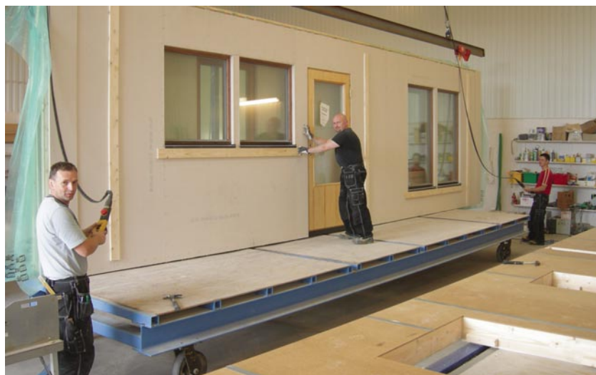
Passive wall complete with insulation and triple glazed windows ready to be shipped from Scandinavian Homes factory in Sweden to a site in Ireland
